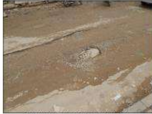
Pavement damage due to sewer line
