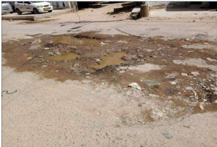
Figure 1-8 Existing Pavement Condition at Saudabad Chowrangi to Urdu Chowk Road
