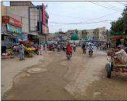
Pavement damage due to sewer line crossing
