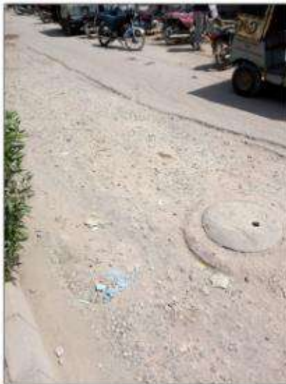
One side of road damaged due to sewer work through-out
