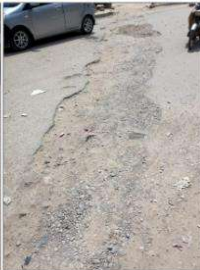
Road damage due to sewer crossing at different locations
