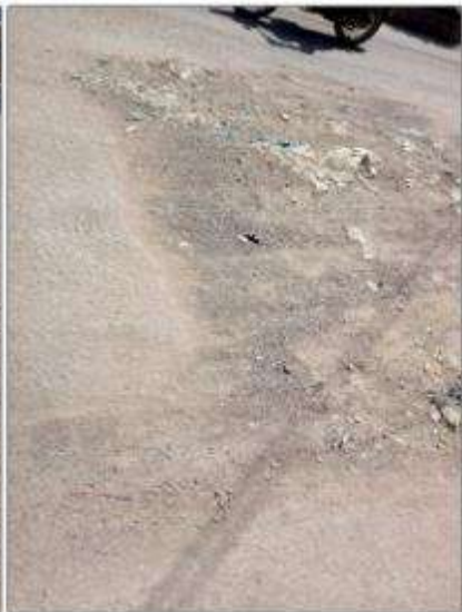
Road damage due to water connection at different locations
