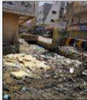
Nullah choked due to garbage at CH: 1+950
