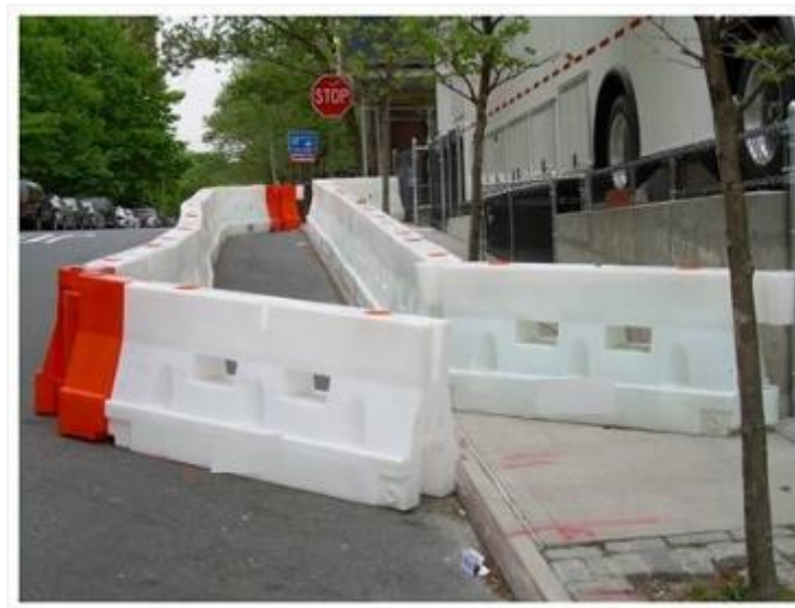
Figure 45: Hard barricade for construction site along the road with access to pedestrian
